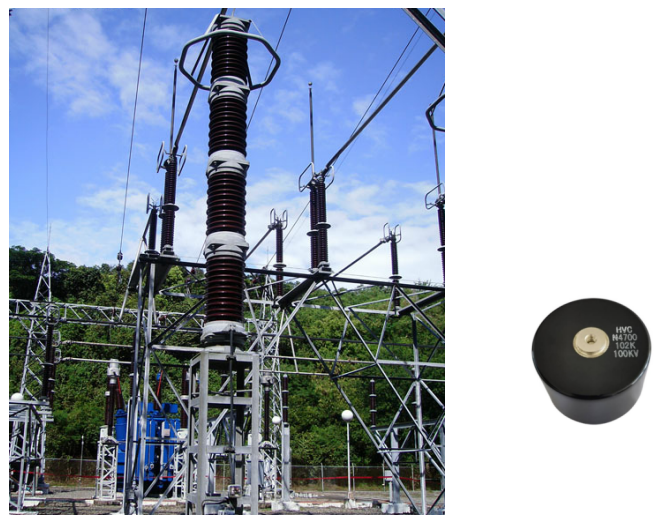
Power Electronic Equipment
